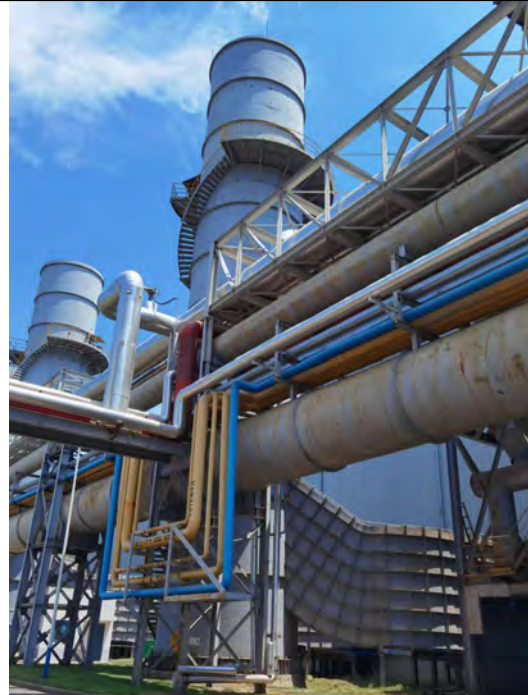
1#精炼炉废气排气筒
