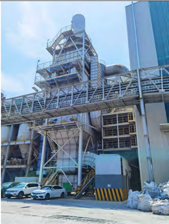
1#湿电除尘废气排气筒
